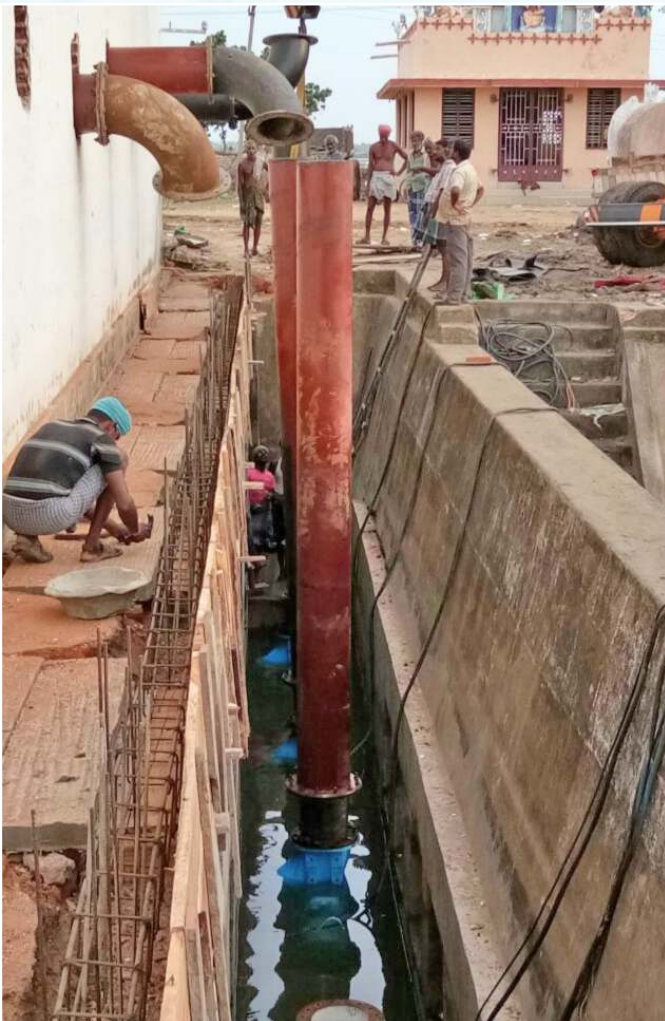
Work on Removal of Old Suction pipes & Installation of New Pumping Machinery
